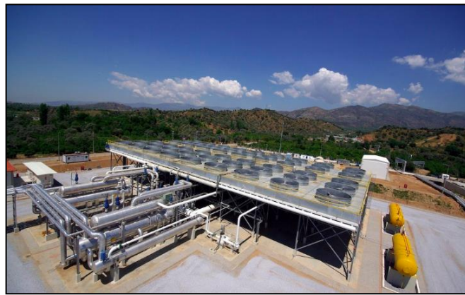
Fig.2. An example for air-cooled type ORC binary power plant in Western Anatolia (Source: ORMAT website).
