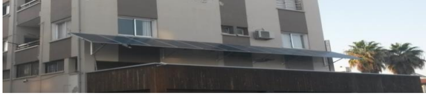
Fig. 1. The picture of the installation.
